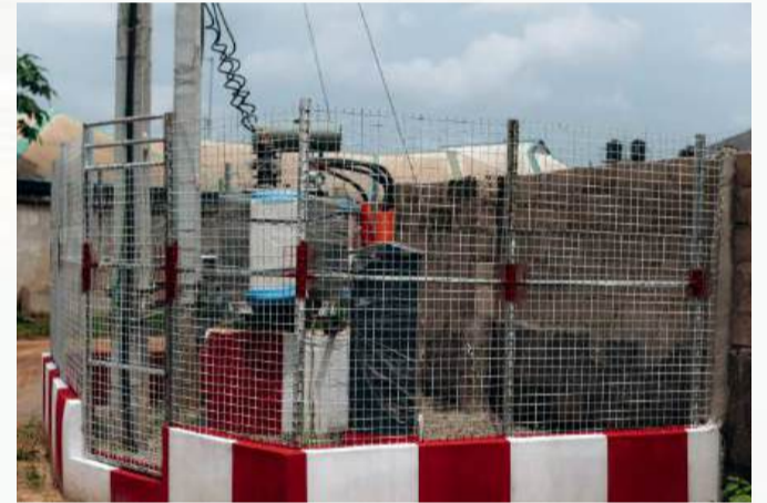
Rural Electrification projects with distribution of transformers in Mbodo Community, Ikwerre LGA
