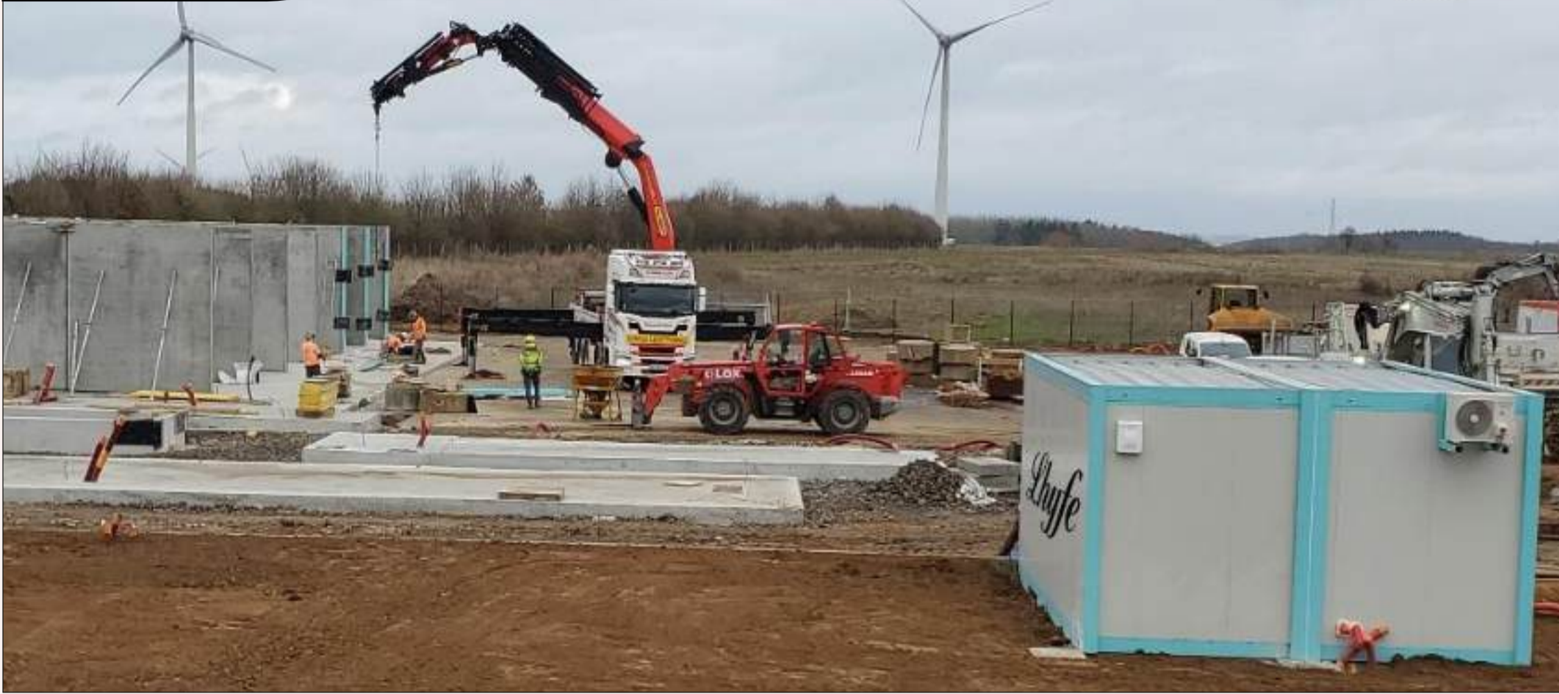
Image: civil engineering work in progress at the Lhyfe site in Croixrault (France)
