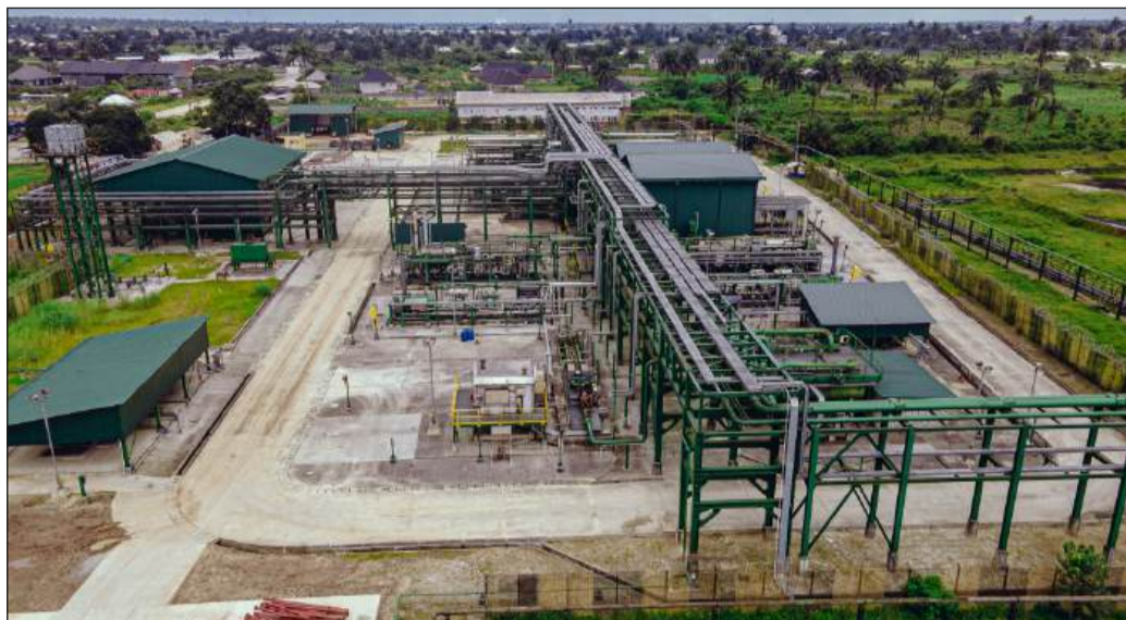
Agbada Non-Associated Gas Plant
