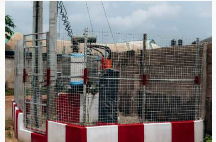
Rural Electrification projects with distribution of transformers in Mbodo Community, Ikwerre LGA
